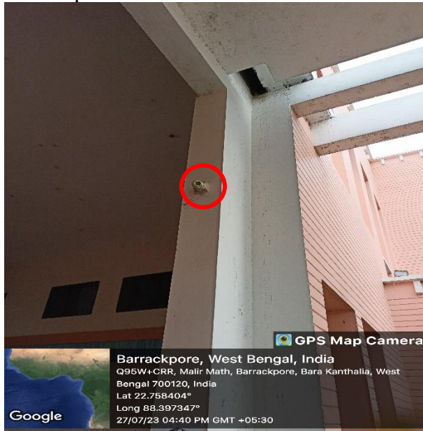
CCTV In Entrance
